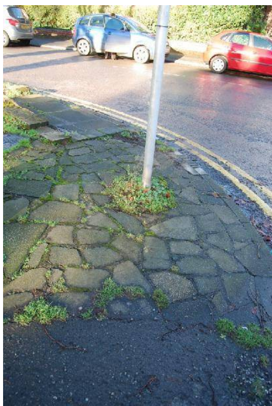
Uneven pavement at The Green
