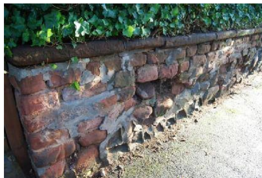
Historic sandstone wall – note decay caused in part by cement pointing
