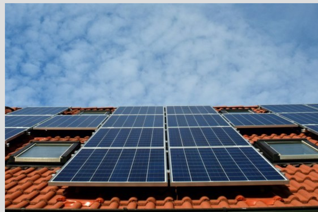
Figure 23: Solar Panels photo credit: Worcestershire County Council
