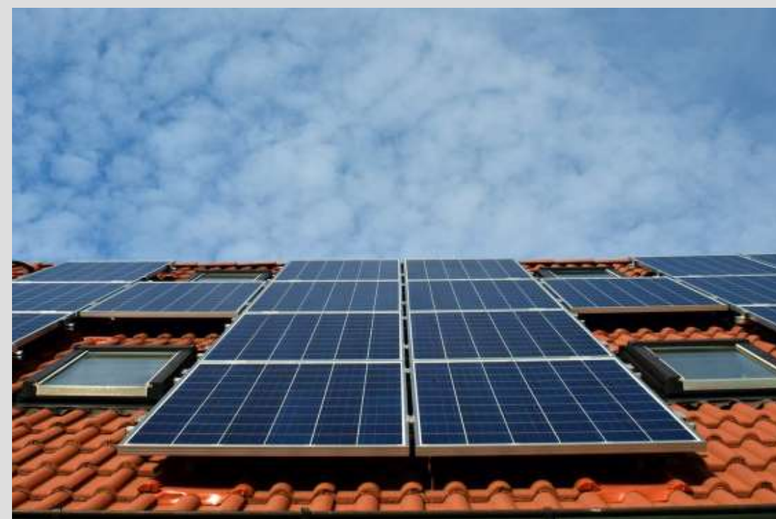
Figure 23: Solar Panels photo credit: Worcestershire County Council
