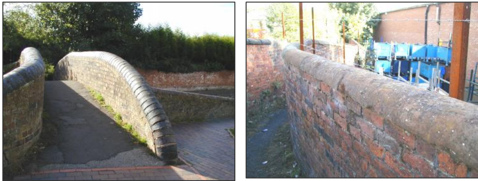
Walls with traditional semi-circular blue brick coping (left) and sandstone coping (right)
