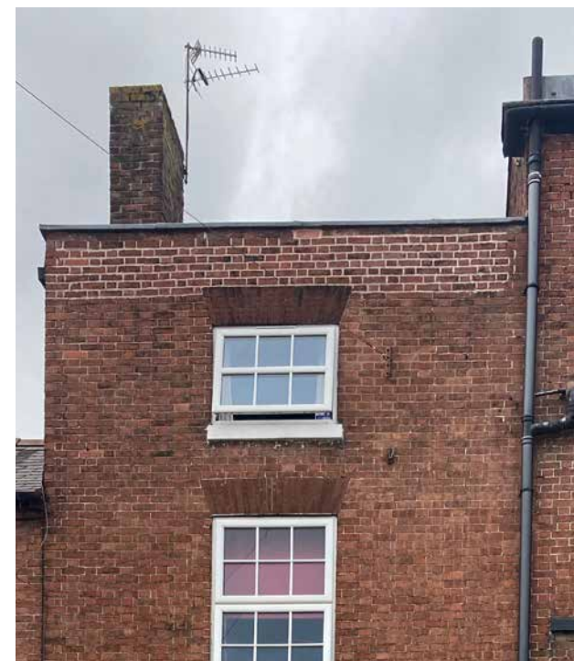
7.1 The use of inappropriate modern windows harms the appearance of buildings
